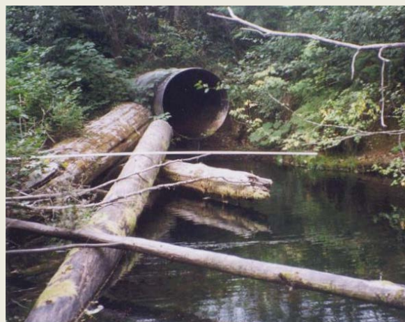
Culverts can act as barriers to fish passage
